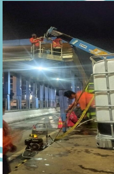
Gambar 3. 10 Maintenance Gerbang Tol
