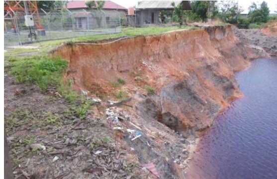
Figure 2. Slope condition after eroded
