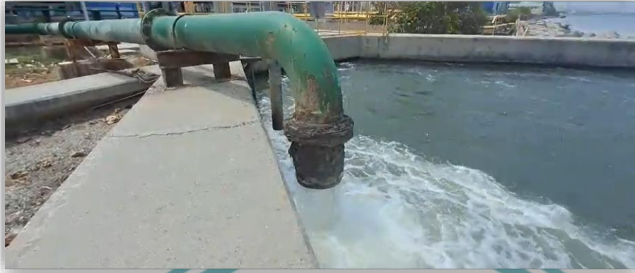
Gambar 1.1 Brine Blowdown Output Line
