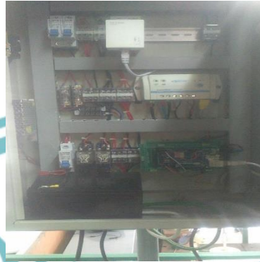
Foto 2. Internal Panel PJU
