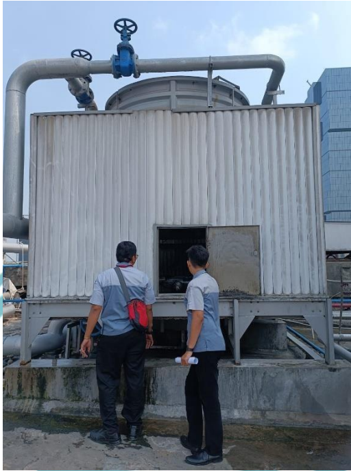
Lampiran 3. Pengecekan Level Air Cooling Tower
