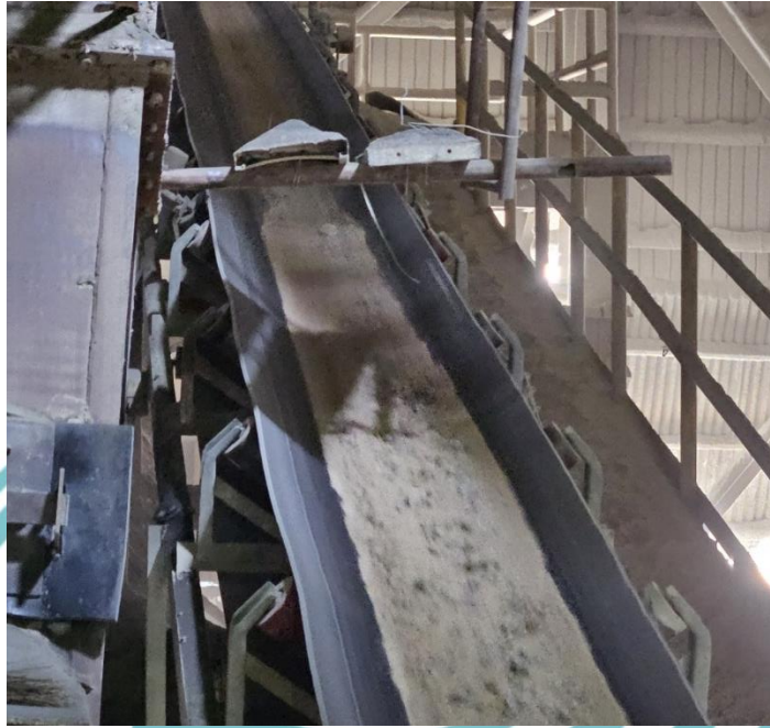
Gambar 3.12 Belt Conveyor Gypsum
