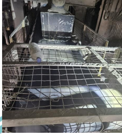
Gambar 3.43 Kelalaian di area Belt Conveyor
