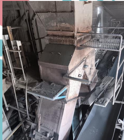
Gambar 3.32 Gate Two Way Chute
