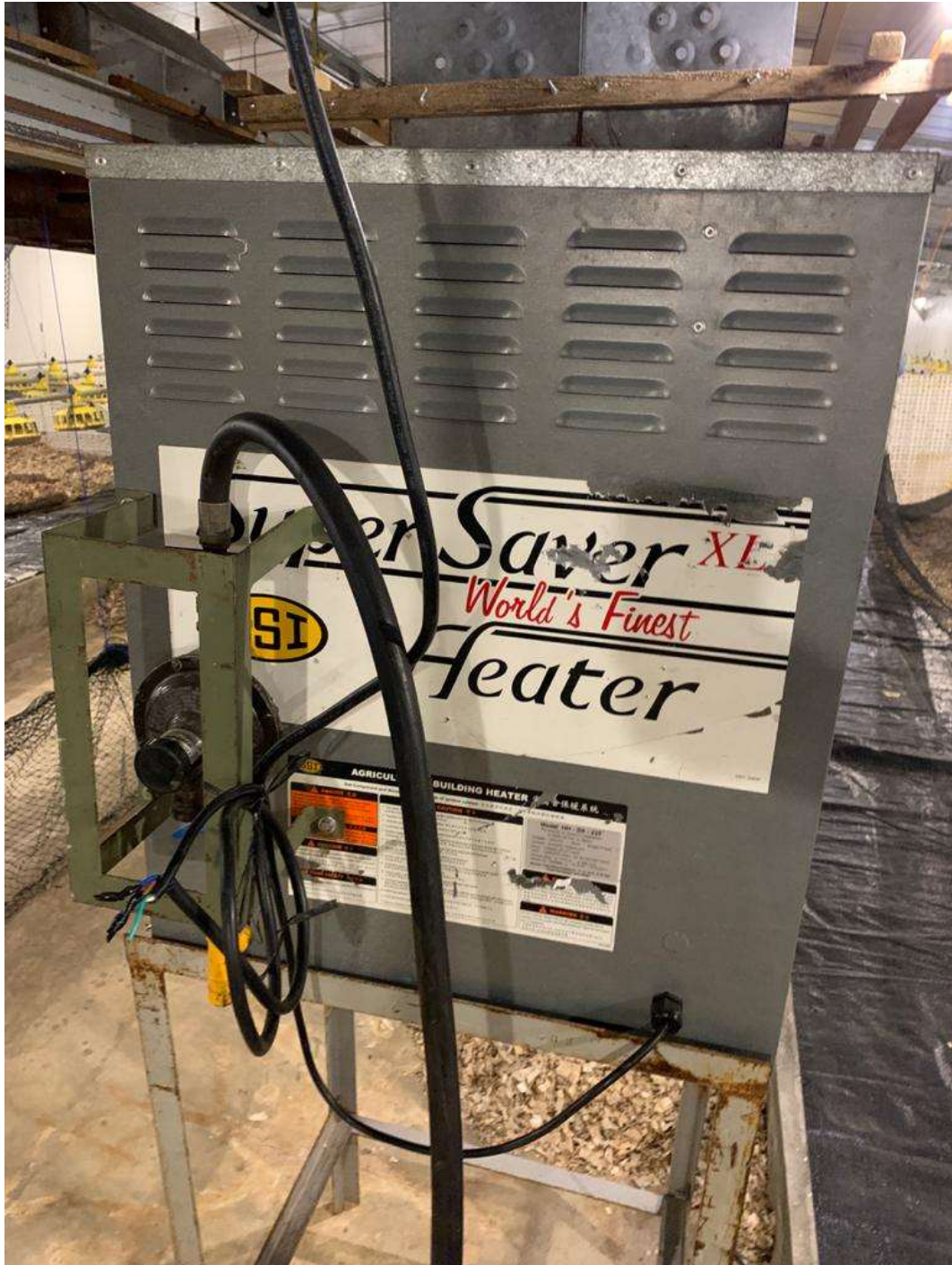
Gambar L 2 Heater Tampak Belakang
