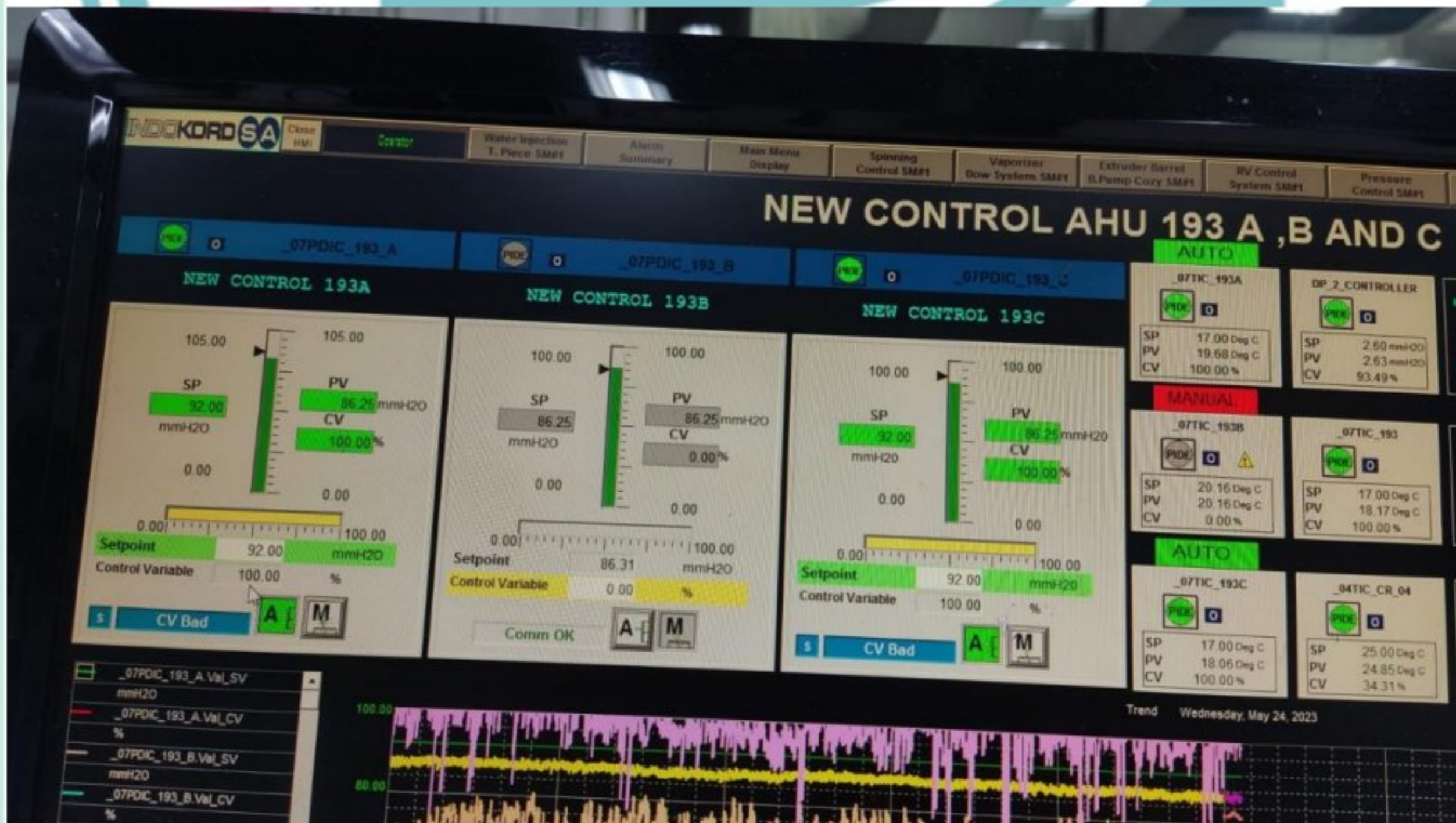
Lampiran 2 Pengoperasian mesin AHU
