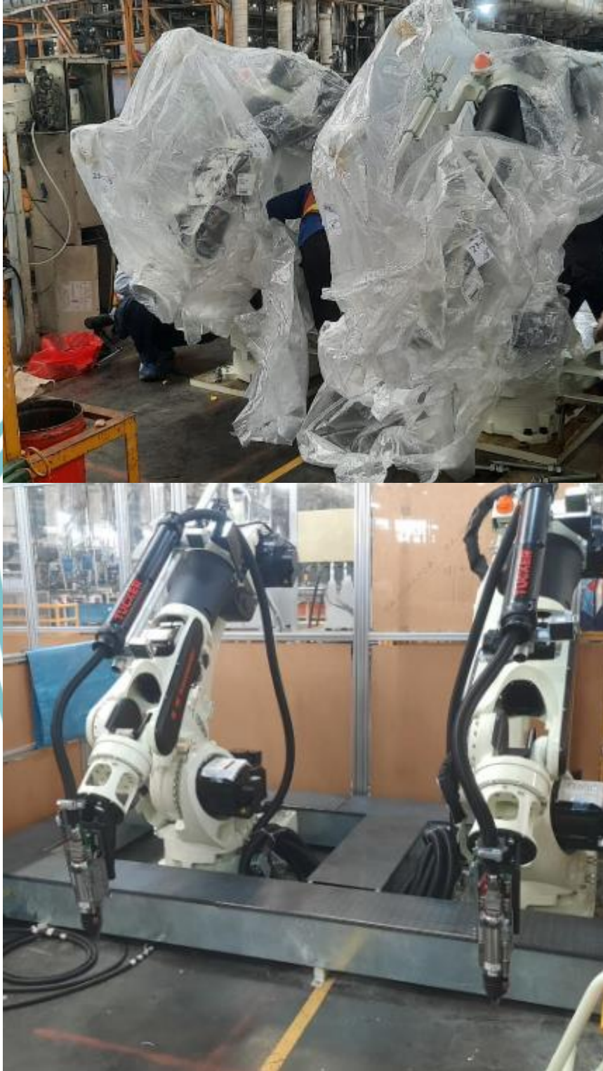
Lampiran 3. Instalasi Robot
