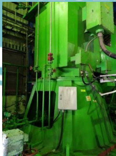
Gambar 3.24 MCWP main cooling water pump
