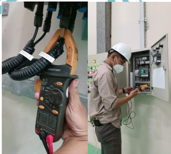
Commisioning PLTS On-Grid di Tower Bank Danamon
